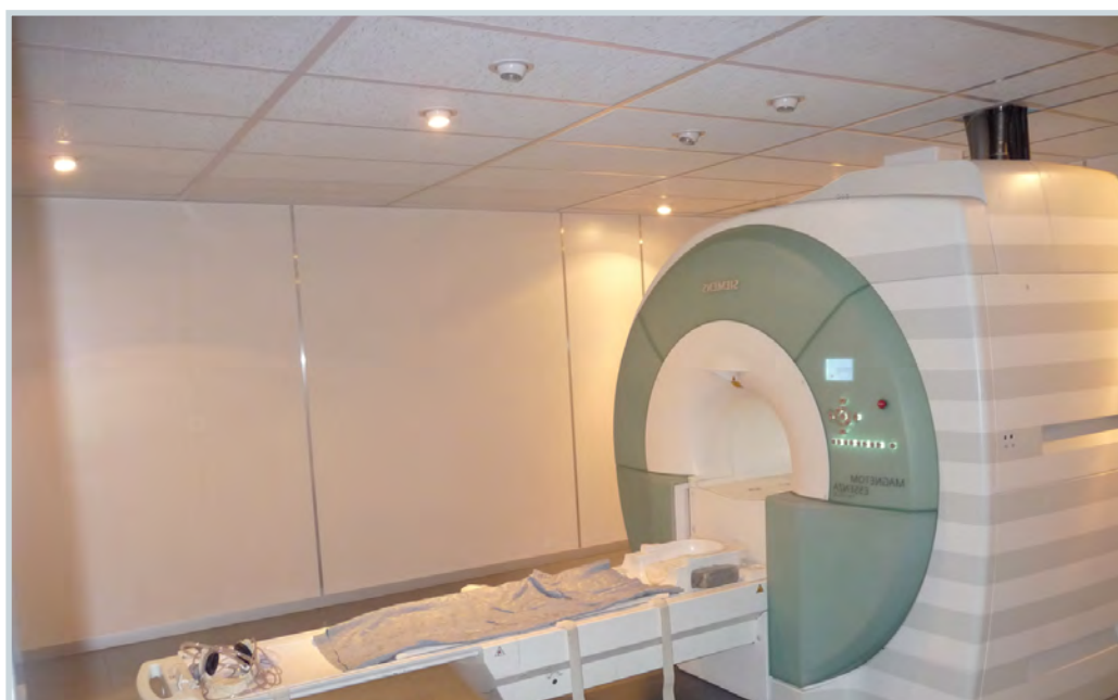
MRI equipment at Cancer Hospital
