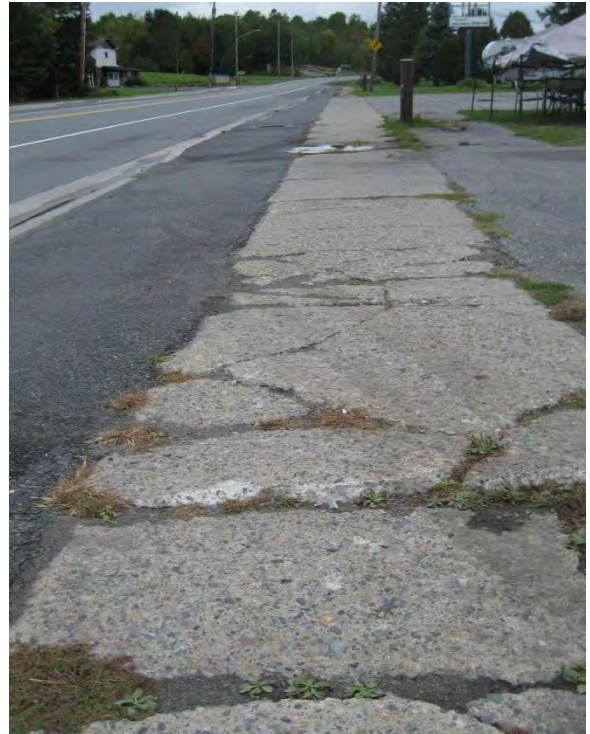
Sidewalks that are not level, such as this one on King Street, may act as barriers to access for people who use mobility aids.
