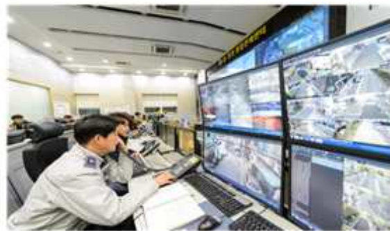
CCTV integrated control tower
